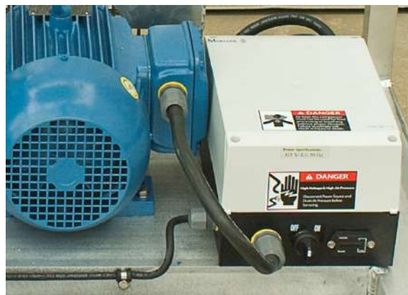
Electric Motor Power Switch and Tach.
