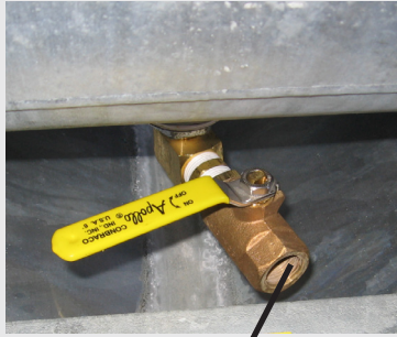
Mixing Tank Drain
