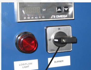
Burner On/Off Switch
